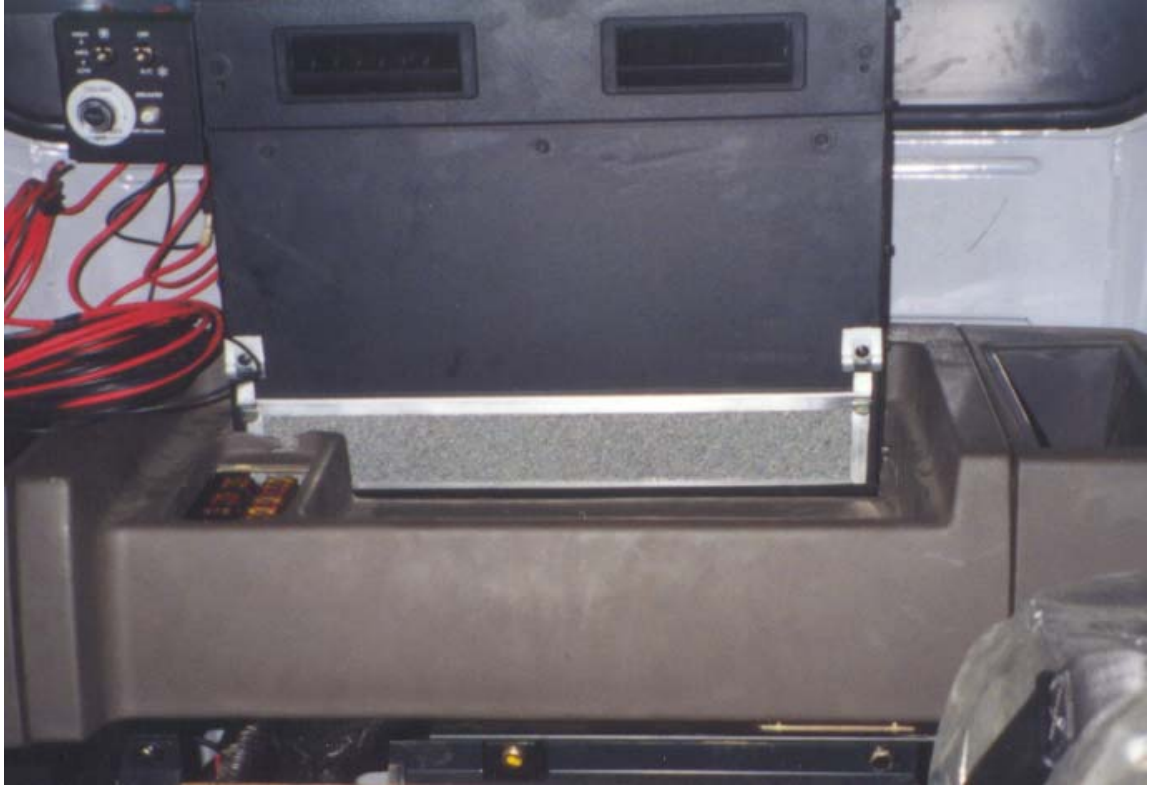
Evaporator in place on back wall of cab. Note that it extends above the lower window line.
