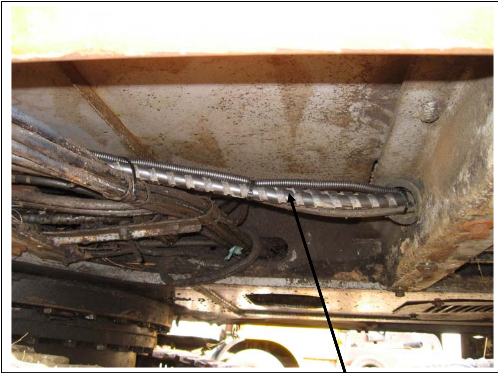
Hoses and wiring running from the radiator compartment forward towards the cab area.
